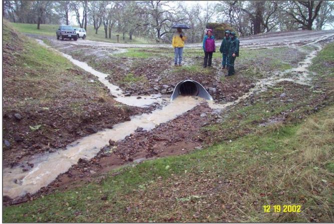
Image 1. Road hydrologically connected to stream and delivering chronic sediment (photo provided by: William Weaver, Pacific Watershed Associates)
